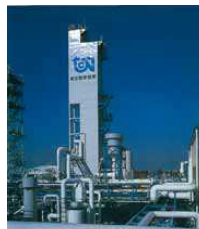
Air separation plant (Chiba)
