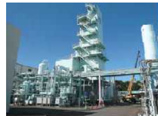
Air separation plant (Aichi)
