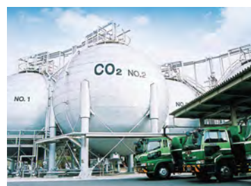
Nippon Ekitan Corporation carbon dioxide gas terminal
