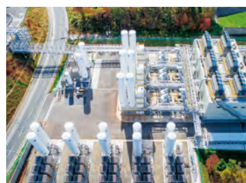
View of the entire facility of Iwate Kurosawajiri Gas Center Corporation
