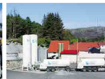
Bulk gas supply facility for an aquaculture facility
