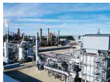
HyCO production facility
