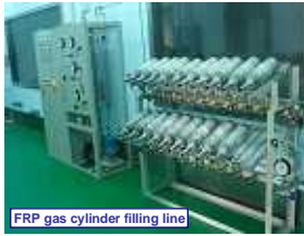
FRP gas cylinder filling line
