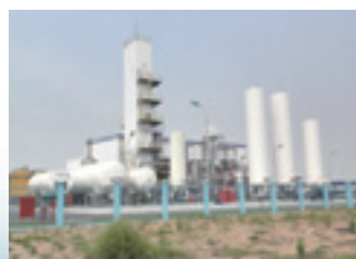
Northern Vietnam Japan Gas Joint Venture Co., Ltd.(ベトナム)
