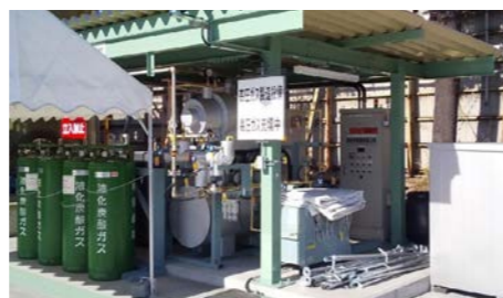
Exterior of the CO 2 liquefaction system
