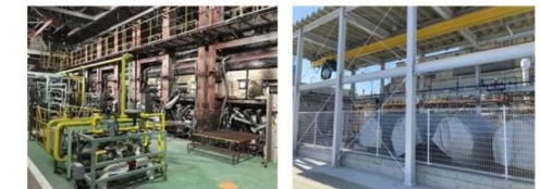
Glass Melting Furnace
